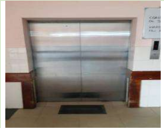
The lift share with the 1 st and 2 nd floor of proposed construction site
